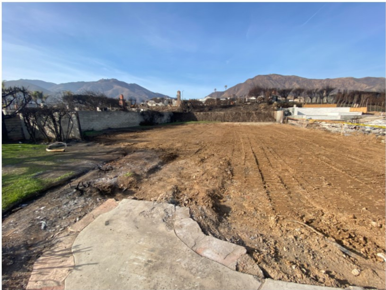
Picture 3: Example of appropriate level of soil removal and foundation clearance (Palisades Fire 2025). Erosion Control will be implemented to prevent sediment runoff.
