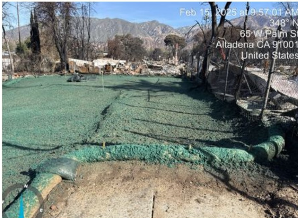
Picture 6: Example of appropriate level of erosion control with hydro-mulch (Eaton Fire 2025). Erosion Control must be implemented to prevent sediment runoff.
