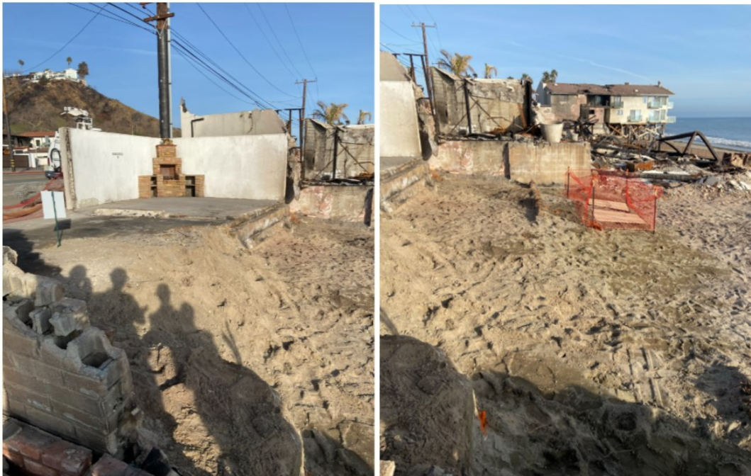
Picture 1 & 2: Example of appropriate level of debris removal and foundation clearance (Palisades Fire 2025). Erosion Control will be implemented to prevent sediment runoff.
