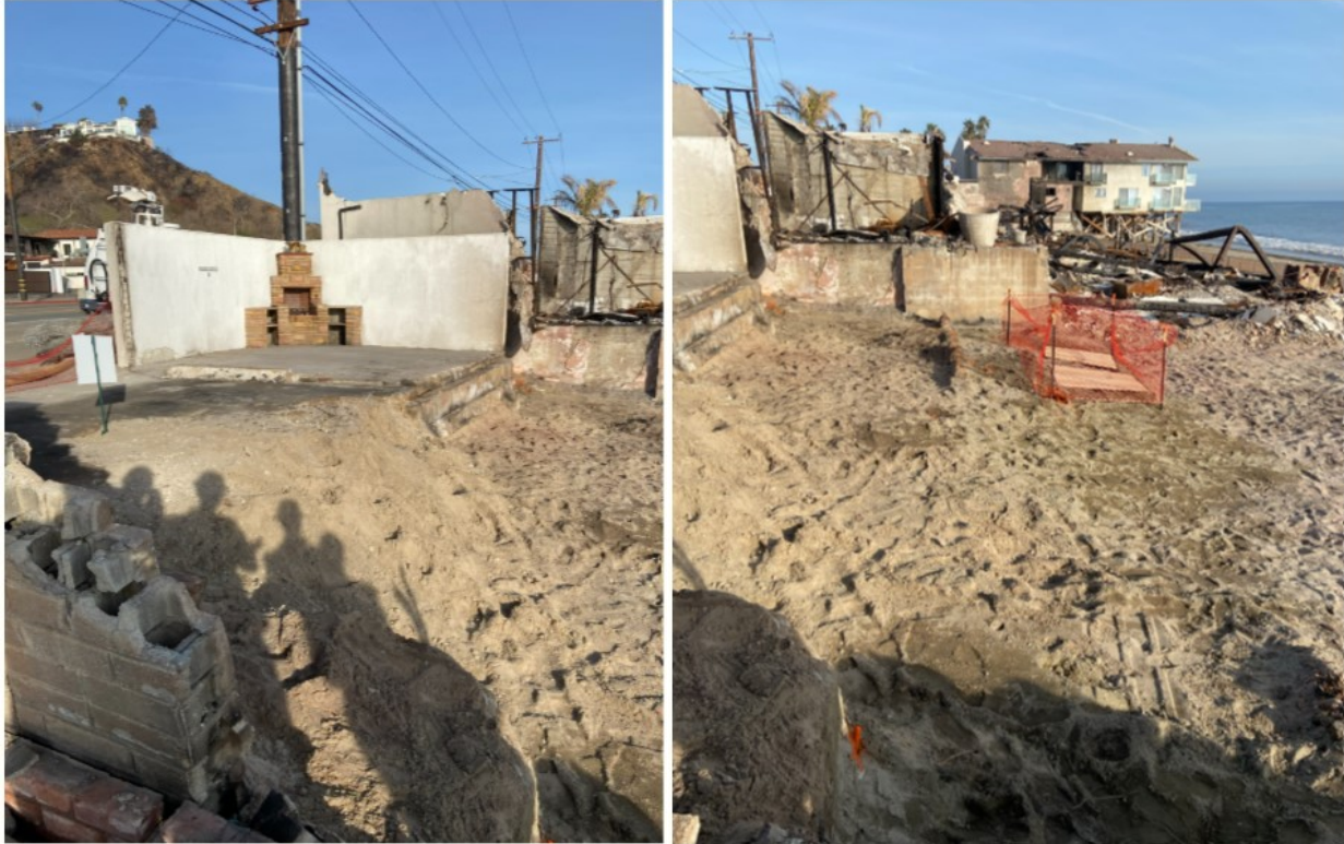
Picture 3 & 4: Example of appropriate level of debris removal and foundation clearance (Palisades Fire 2025). Erosion Control will be implemented to prevent sediment runoff.
