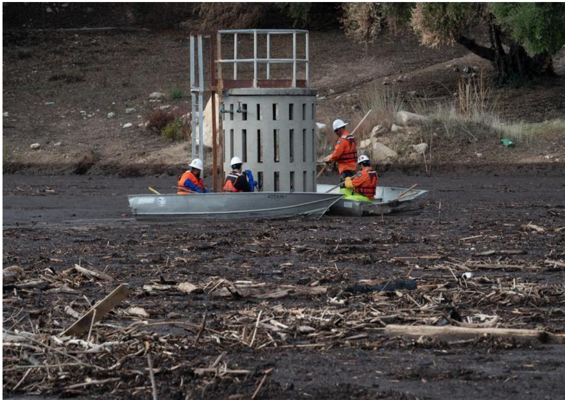
Photograph of post-Eaton Fire debris flow at Rubio Wash Dam
