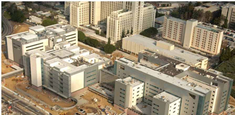
Above is an aerial photo of the new LAC+USC Medical Center Replacement Hospital under construction. The new hospital is approximately 1.5 million square feet, and consists of the Outpatient Building, Diagnostic and Treatment Center, Inpatient Tower, and a Central Plant. The Replacement Hospital will open during the 2007-08 fiscal year.
