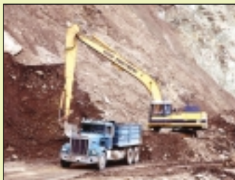
Public Works staff clears landslide on Lake Hughes Road in Angeles National Forest near Santa Clarita following rainstorm.
