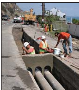
Public Works crews work around the clock to repair a water pipe on Pacific Coast Highway.
