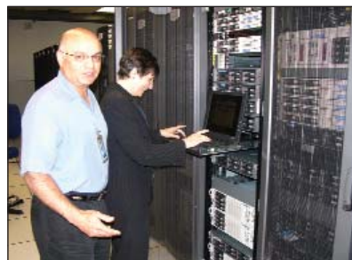
Information technology main server
