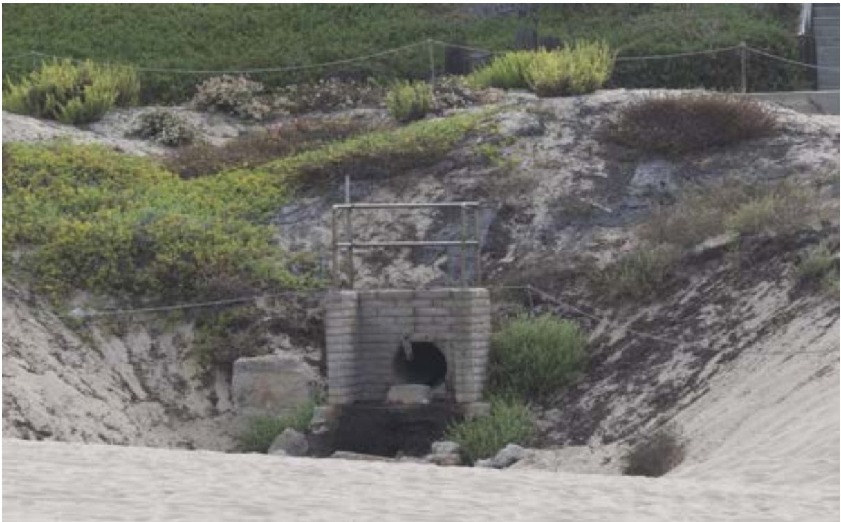
Photograph 16. View culvert outlet directing stormwater flows into back beach. Note developed and disturbed landscape surrounded by the coastal scrub habitat of the Manhattan Beach Dune Restoration site at the Manhattan Beach study area, facing north.
