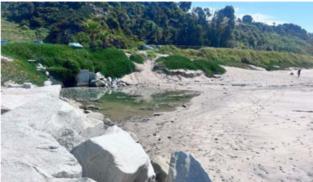
Photograph 8. View of culvert outlet directing stormwater flows onto the back beach. View of sandy beach, ice plant mats, and developed/disturbed/landscaped landcover types at the Will Rogers State Beach study area, facing east.
