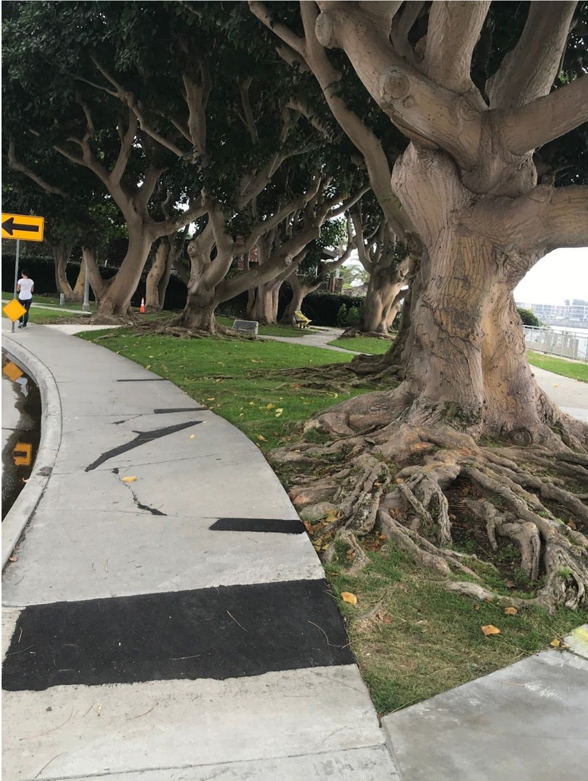
Photo 1 – VM-27, major structural roots causing sidewalk to lift.
