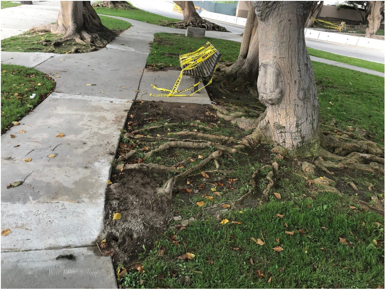
Photo 4 – Tree VM-33 large roots causing lifting and damage to sidewalk.
