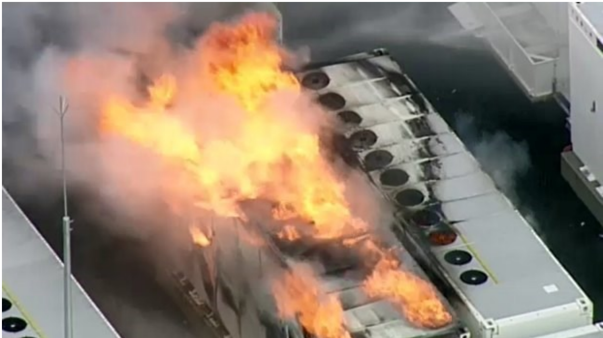
Figure 1. BESS Fire Resulting from a "Thermal Runaway" Event.
