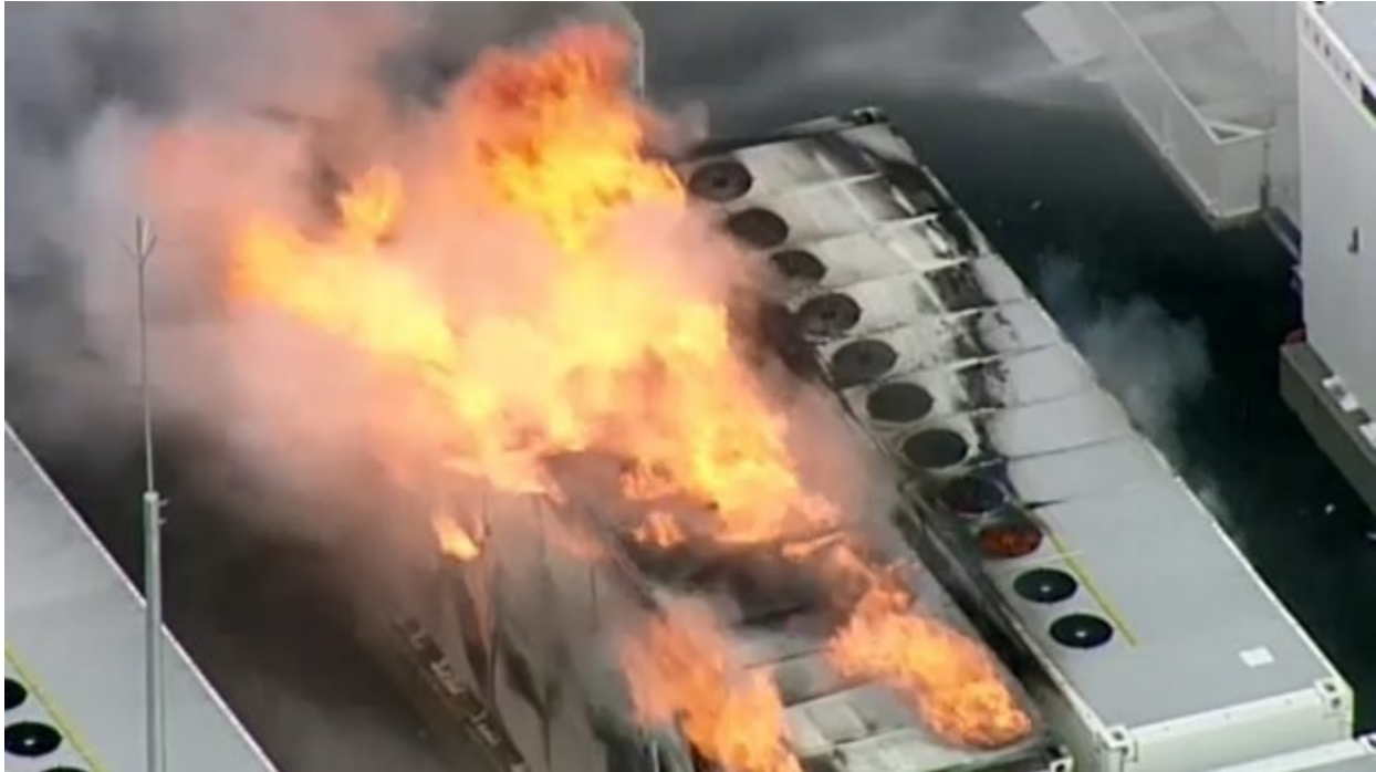
Figure 3. Containerized BESS After Thermal Runaway Initiates.
