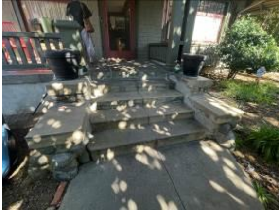
Figure 4. Detail of Entry Porch, Primary Façade (cast concrete steps accented with arroyo stone and cast concrete porch deck) SOURCE: Sapphos Environmental, Inc., 2023
