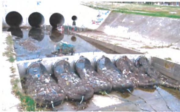
Figure 8. Stormwater Systems – StormX Netting Trash Trap. The picture displays a netting system inside a channel downstream of an outlet
