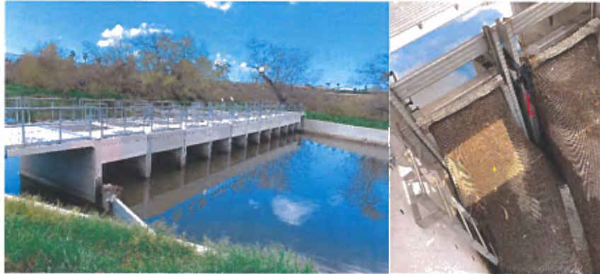
Figure 7. Wilmington Drain Trash Netting System. The picture shows the StormTrap TrashTrap looking downstream in Wilmington Drain (left). These are 5mm drain nets or socks inside the precast chamber (right).
