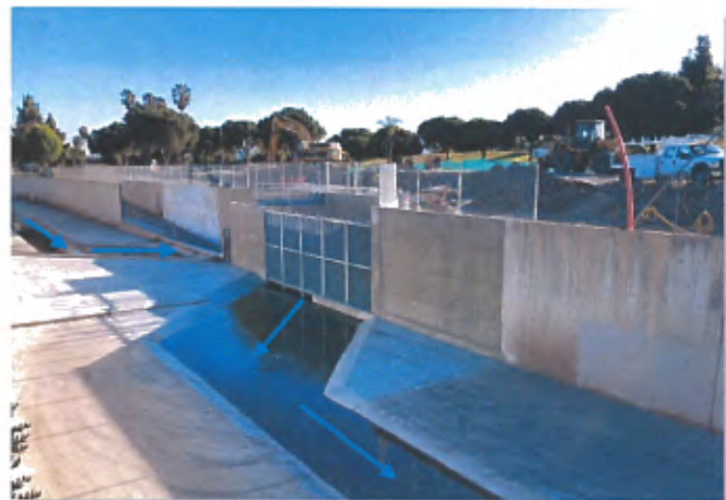
Figure 6. Santa Ana-Delhi (SAD) Diversion Project. This is the SAD Diversion Project in construction looking upstream. The blue arrows show the water and trash path of travel.
