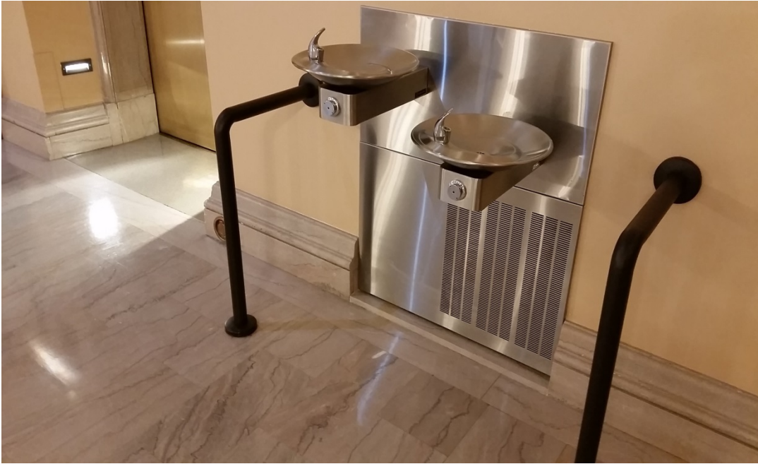
Drinking Fountains – Wheelchair Accessible
