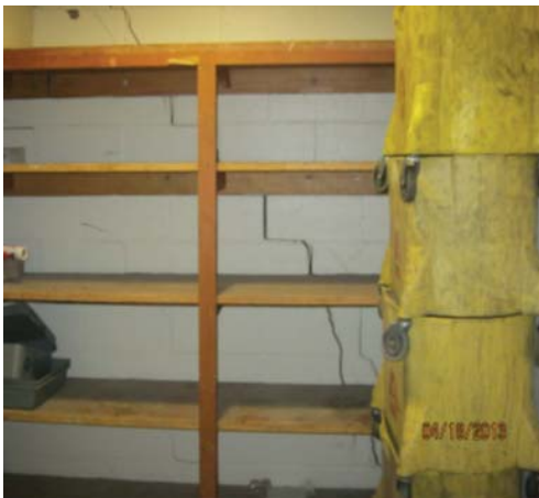
Figure 1.28: Mira Loma Dining Hall Structural Damage
