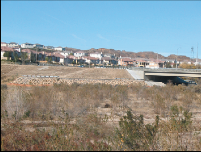
Stabilization at San Francisco Creek at the West Bank (This photo depicts exposed bridge abutment)
