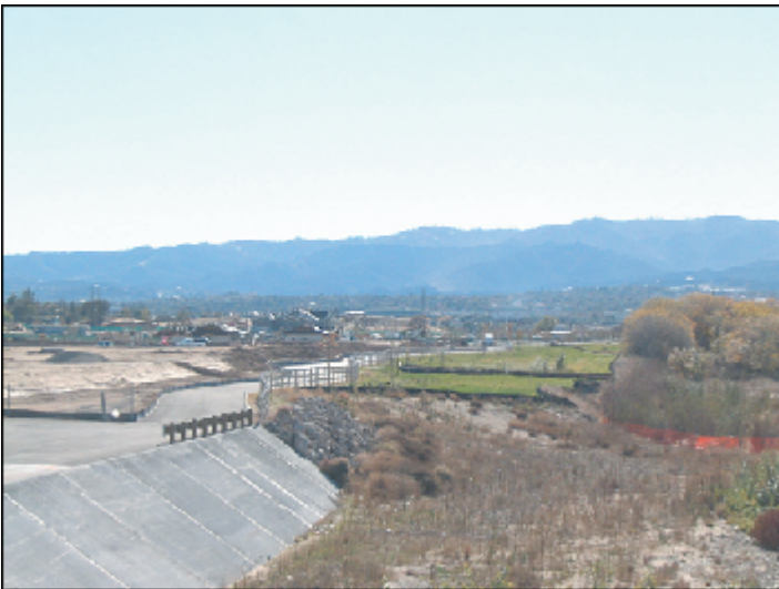
Stabilization at East Bank from Decoro Bridge (This photo depicts River/Buried Bank Stabilization, Upland Preserve and a Trail)
