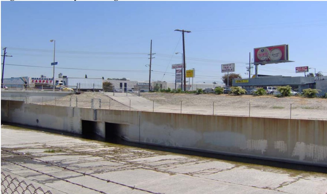
Photograph 6: Tujunga Wash channel (view from west terrace looking northeast) towards Sherman Way – The northern limit of the project in the City of Los Angeles North Hollywood neighborhood
