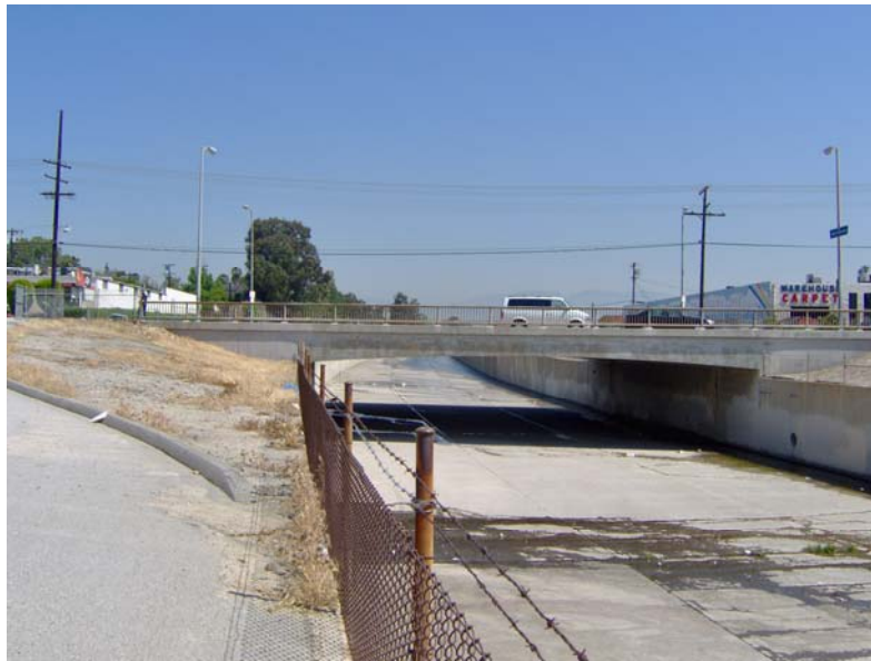
Figure 4: Up Stream Boundary of Tujunga Wash Restoration Project at Sherman Way Bridge
