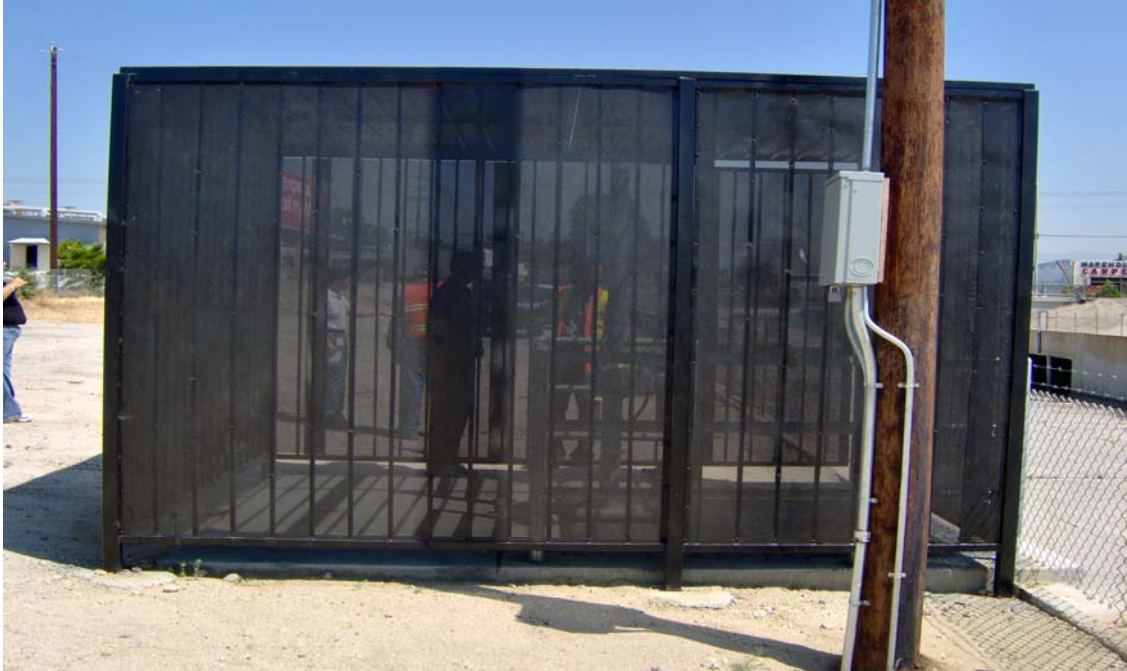
Photograph 12: Intake gate and protective cage looking north (team members provide scale). West side, Tujunga Wash channel near Sherman Way gate.
