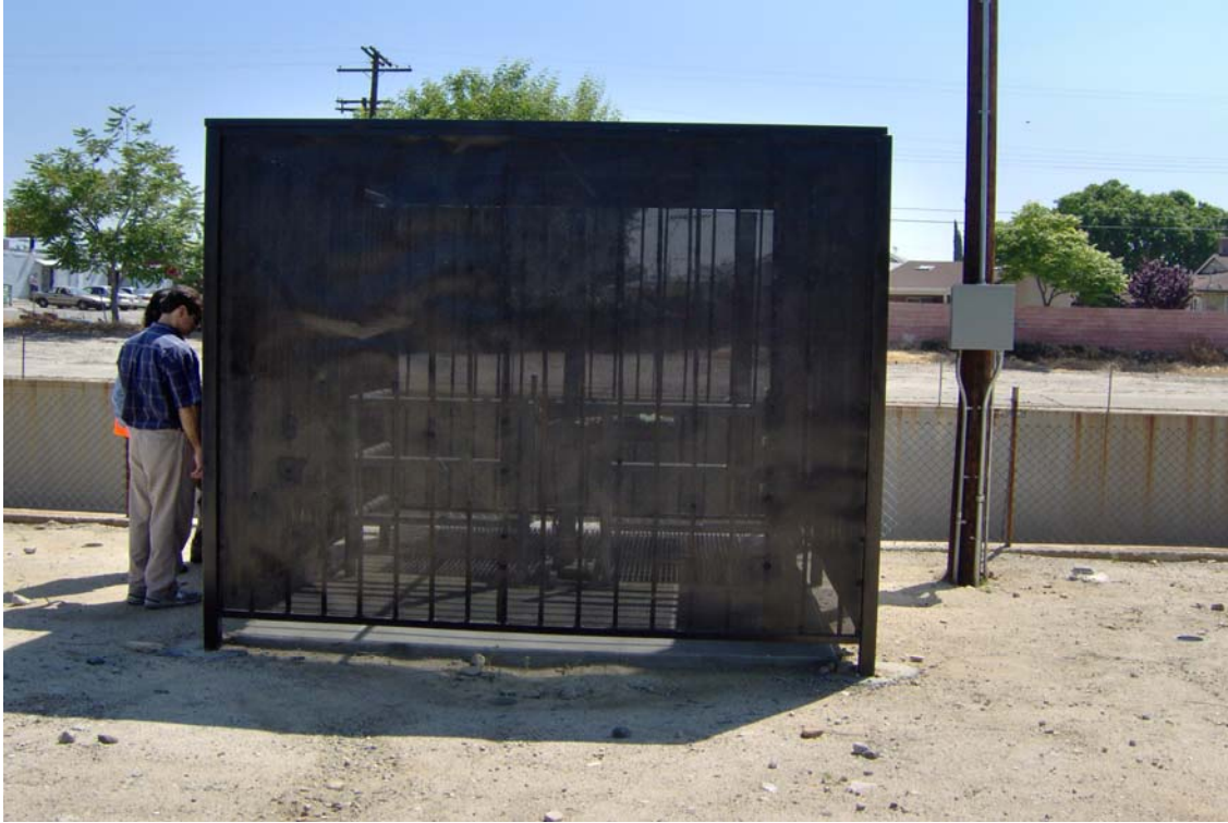
Photograph 11: Newly completed (2005-2006) cage protects gravity-flow intake/slucie gate to provide Tujunga Wash 1134 project with water for the ecosystem restoration component.
