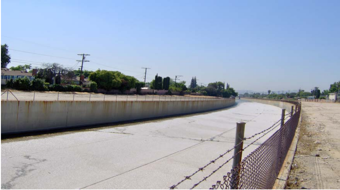
Photograph 13: Downstream view of Tujunga Wash channel from west side (near cage for intake gate). Note existing chain link fence will be replaced (keeping with sponsor's plans for their on-going river restoration) with OMEGA fencing, considered a safer alternative for finished projects.
