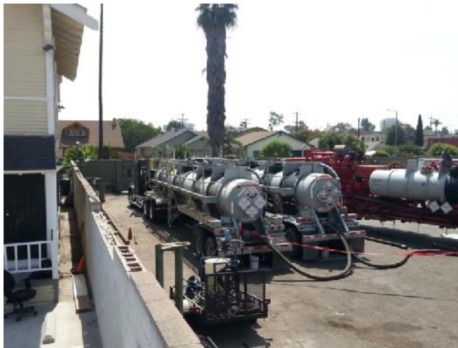
July 15, 2014: Heavy diesel equipment including two tanker trucks behind red DANGER tape sit idling outside bedroom windows at FMOG's Jefferson Drill Site.
