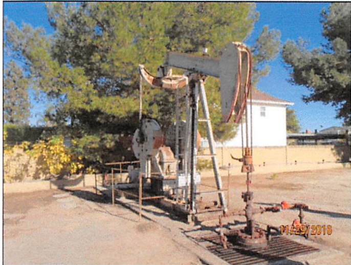
Image: Pump jack located within feet of homes at Brea Canon Lease.
