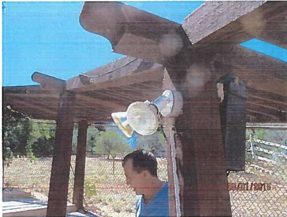
Picture 6 Unshielded Exterior Flood Lights
