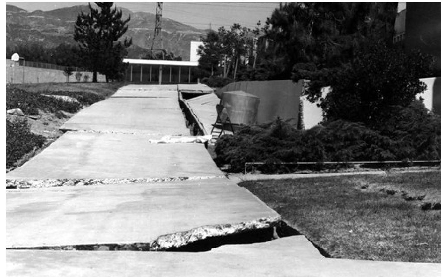
Damage to Sylmar/San Fernando Juvenile Hall following the 1971 earthquake
