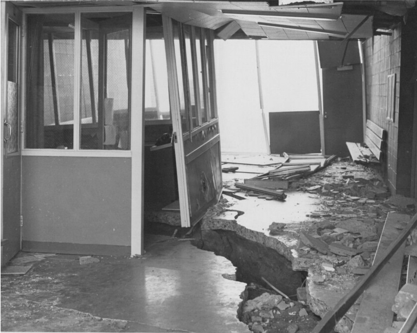
Damage to Sylmar/San Fernando Juvenile Hall following the 1971 earthquake
