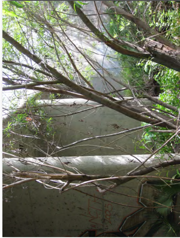
4. Looking northeast at the entrance of the triple box culverts from the downstream side.
