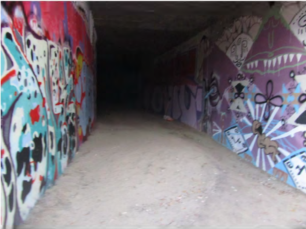
Photograph 4- Sediment accumulation in the eastern cell of the triple concrete box culvert.
