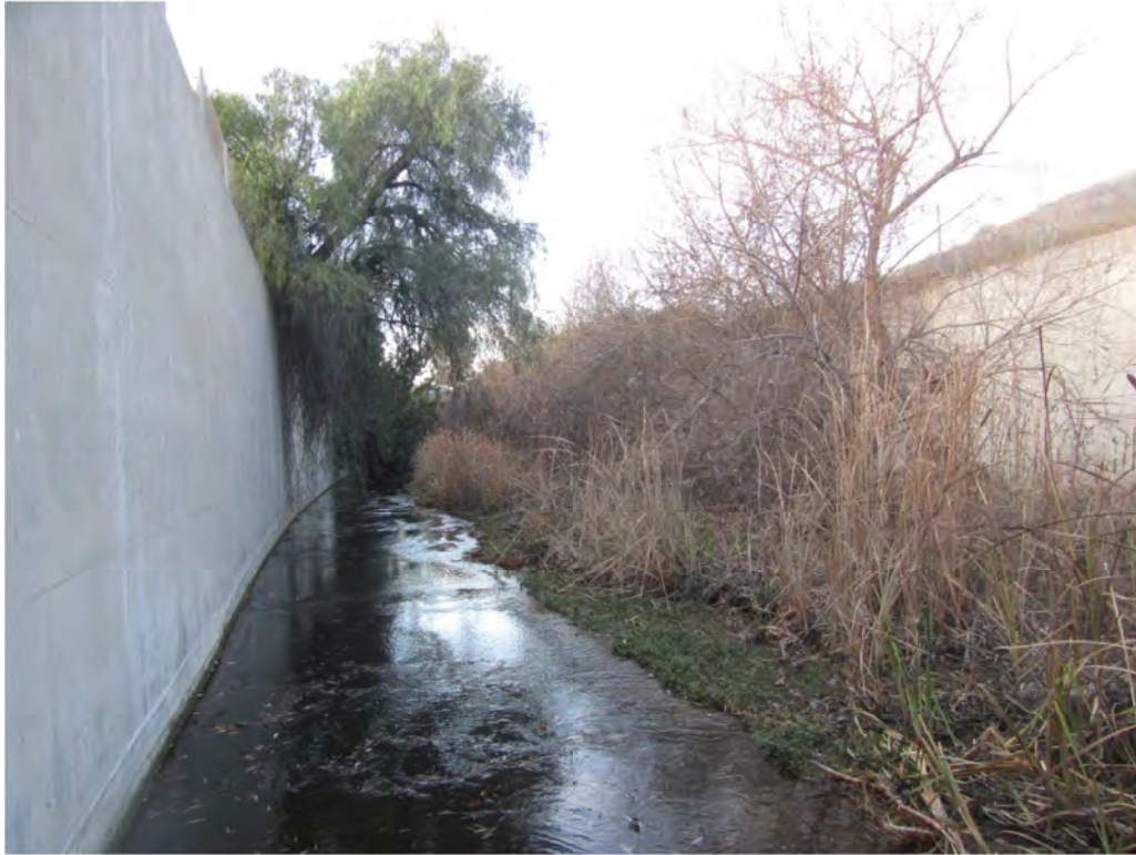
Photograph 5- North of U.S. Route 101, looking at the low flow channel along the southern wall of the open culvert, and the accumulated sediment on the northern wall of the open culvert.
