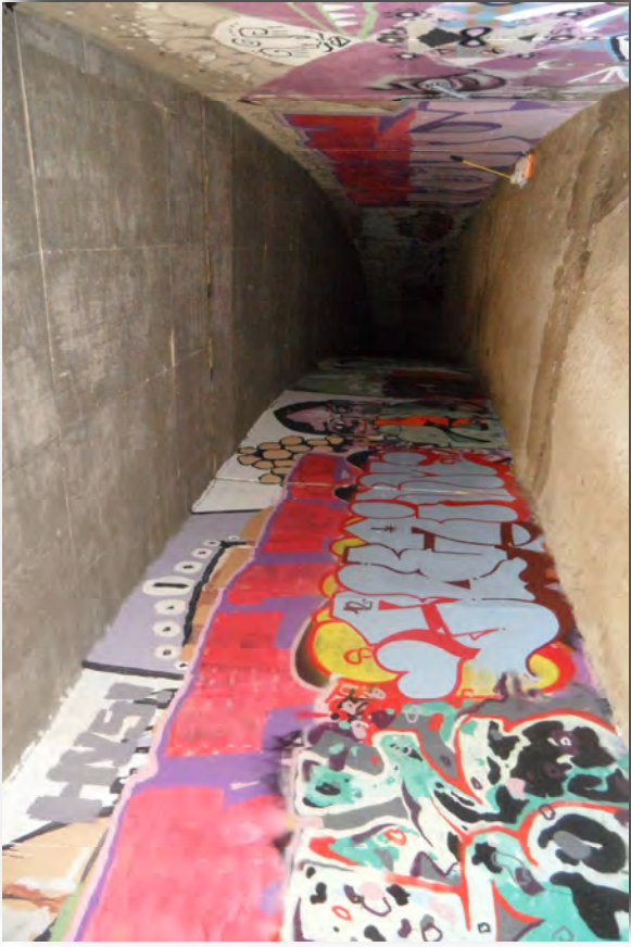
7. Looking south from the northern entrance into the western barrel of culverts.
