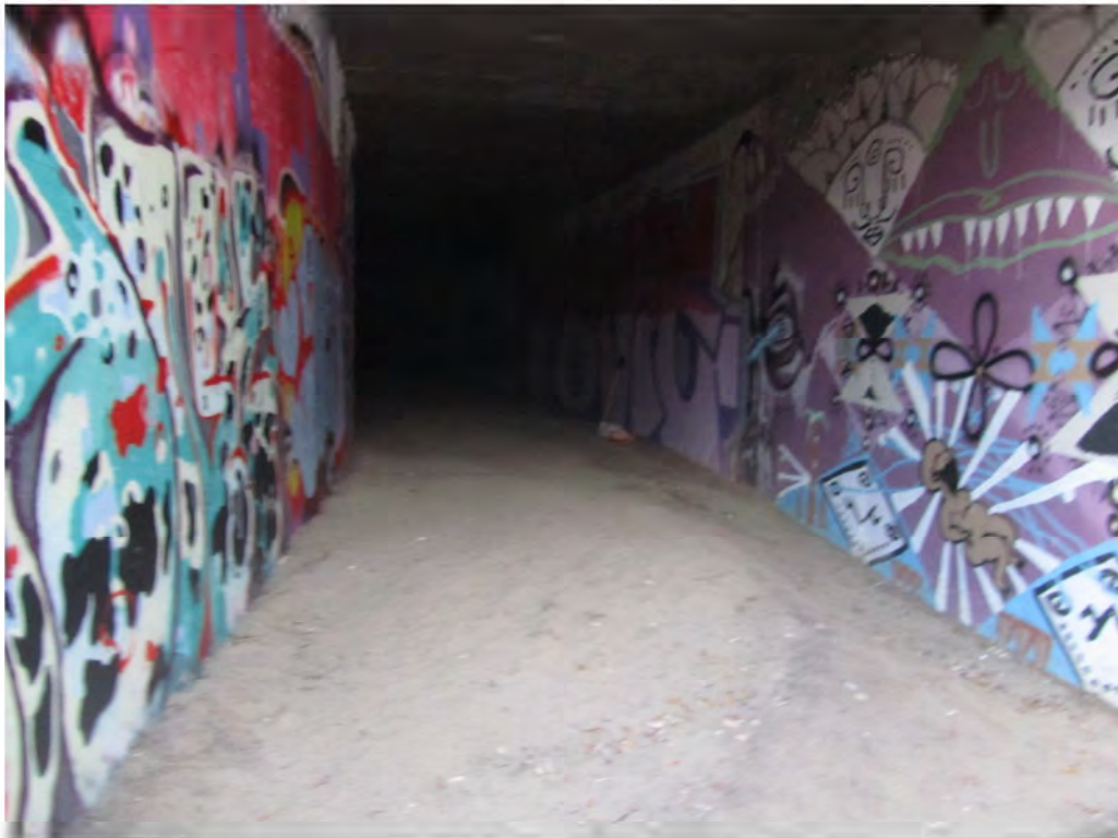
Photograph 4- Sediment accumulation in the eastern cell of the triple concrete box culvert.
