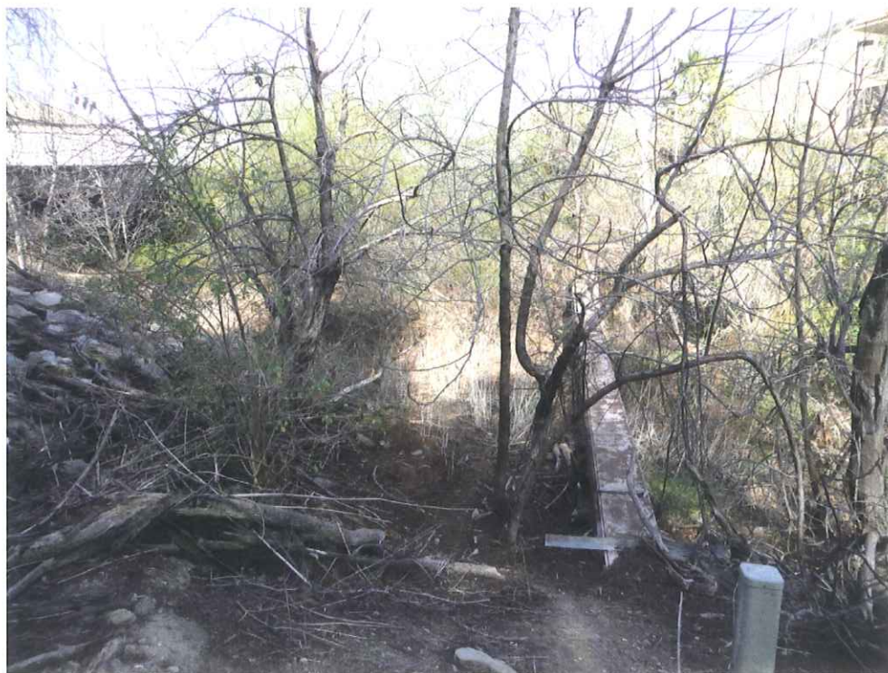
Photograph 8- Large steel beam crossing over Las Virgenes Creek on the right. Riprap stabilized bank on the left.
