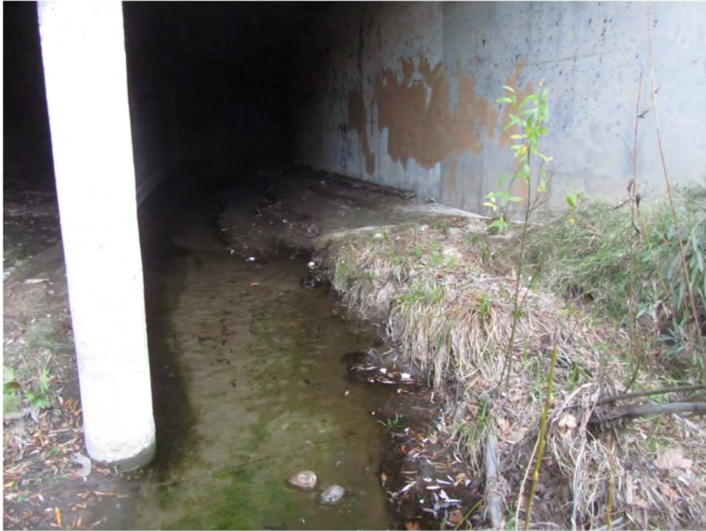
Photograph 3- Low flow channel flowing through the western cell of the triple concrete box culvert under U.S. Route 101.
