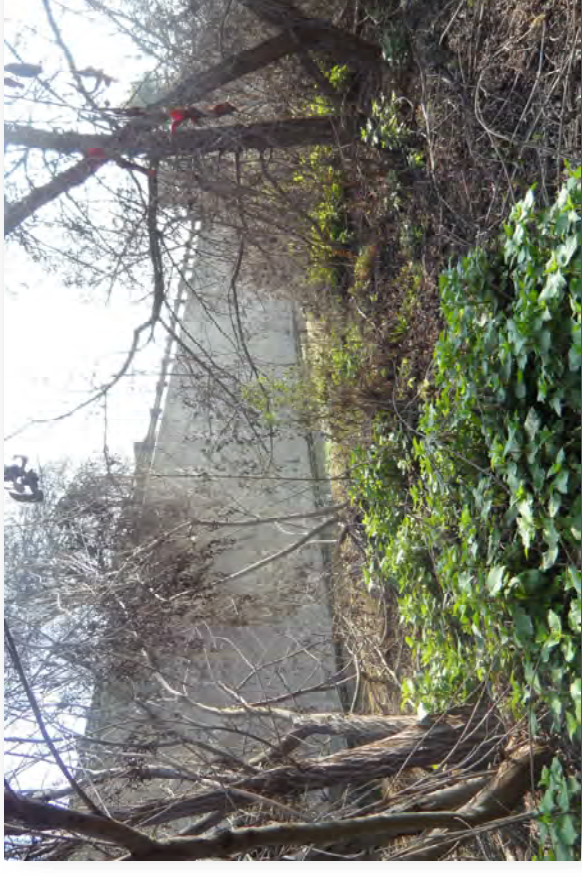
6. Looking north from the northerly entrance of the western barrel of the culverts.
