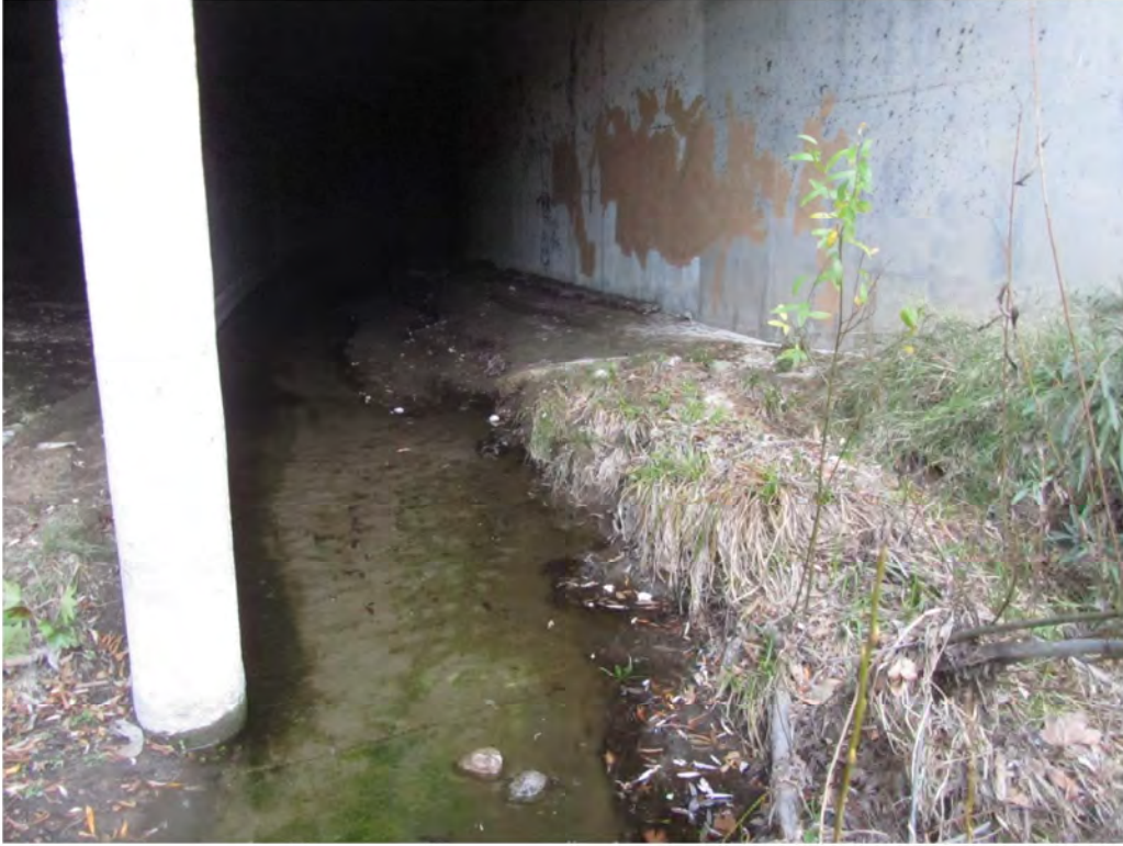
Photograph 3- Low flow channel flowing through the western cell of the triple concrete box culvert under U.S. Route 101.
