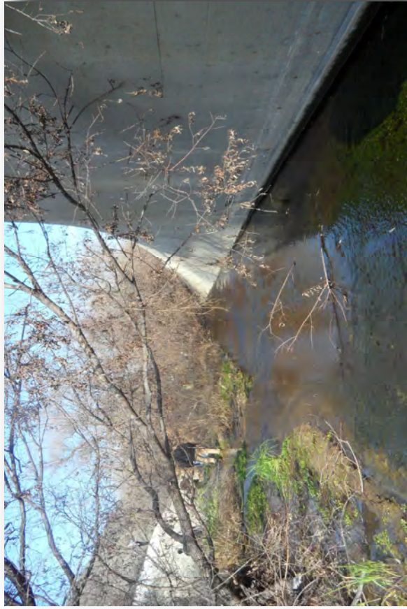
10. Looking upstream at the transition from the concrete channel to the natural channel.
