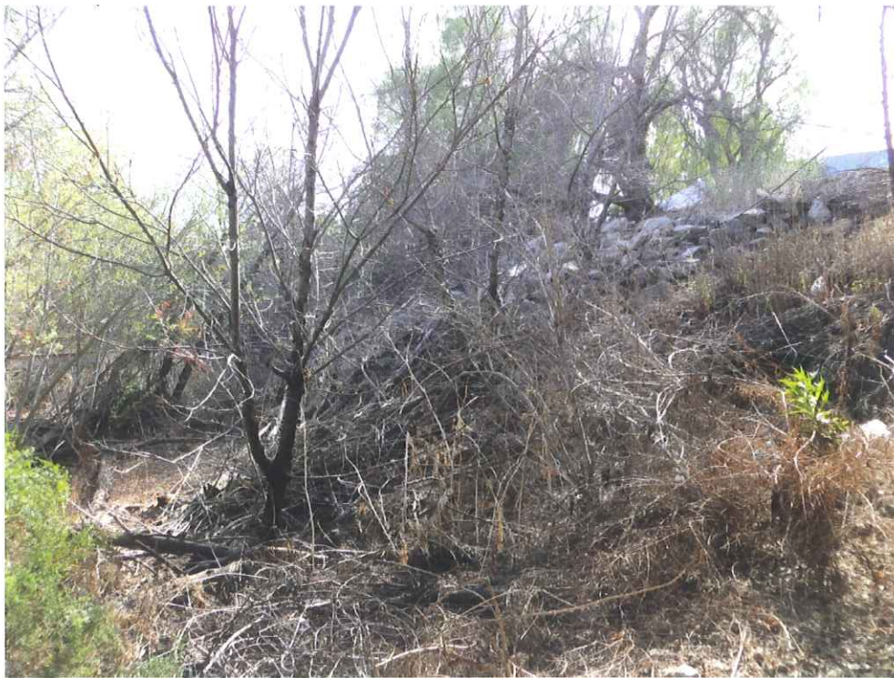
Photograph 6- Vegetation growing up through the open riprap on western bank.
