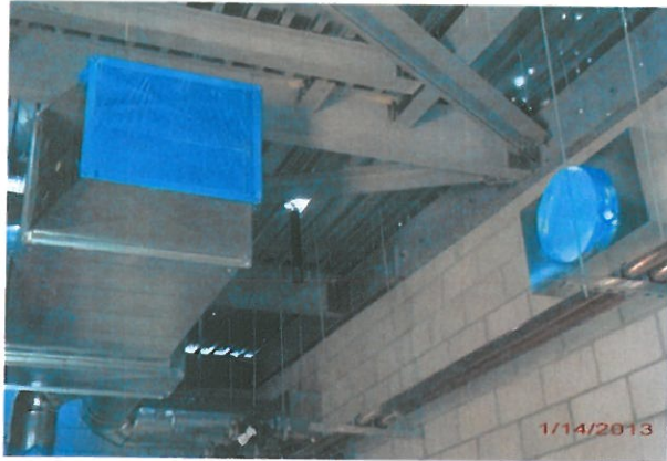
HVAC Duct Opening Sealed during Construction
