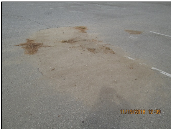
(Photo 9) “Sink-hole” in parking area along eastern boundary, approximately 135 feet south of the northeast corner of the property. Backfilled with soil from unknown source. Cause and volume unknown.
