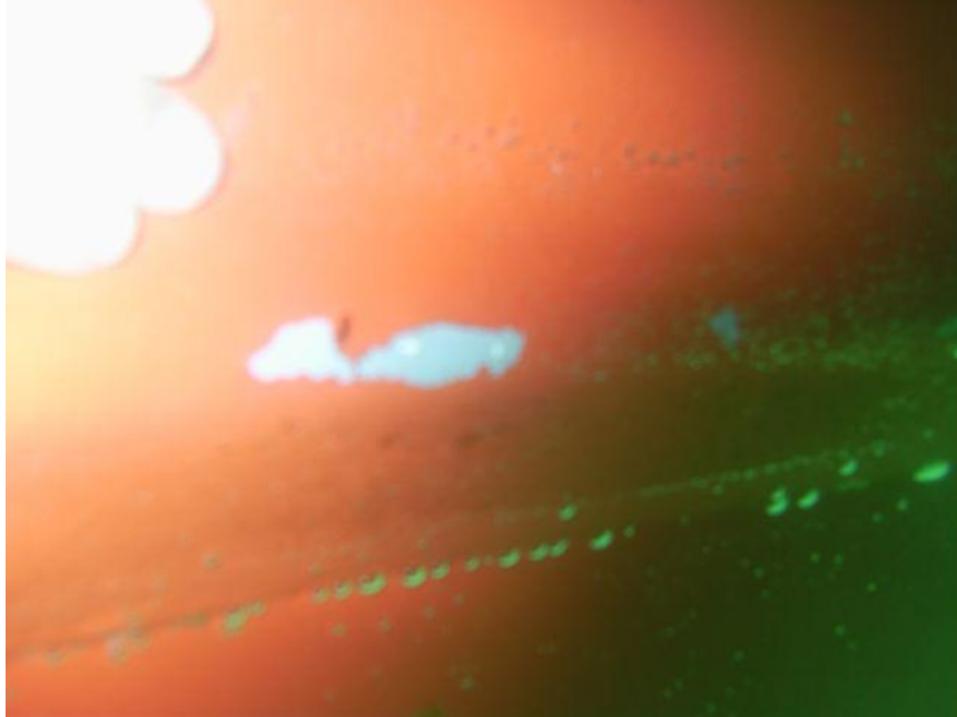
Figure 5-24. Underwater Picture of Peeling Paint
