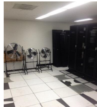
Aging equipment in aging facilities
