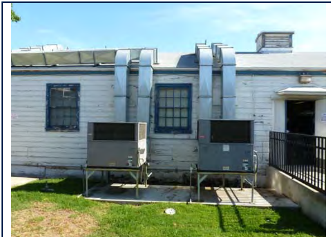
South elevation, HVAC ducts. 6/11/13.
