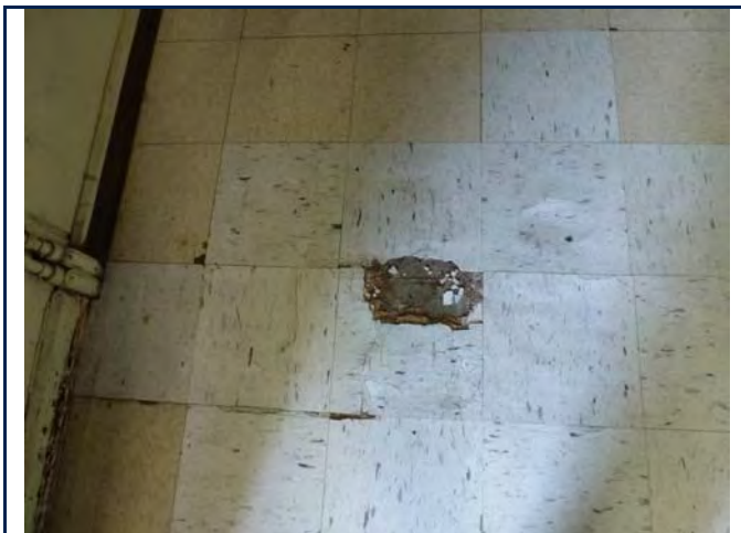
Interior, floor damage. 6/11/13.
