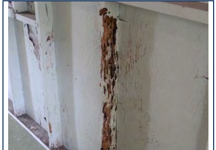
Interior, severe termite damage. 6/11/13.
