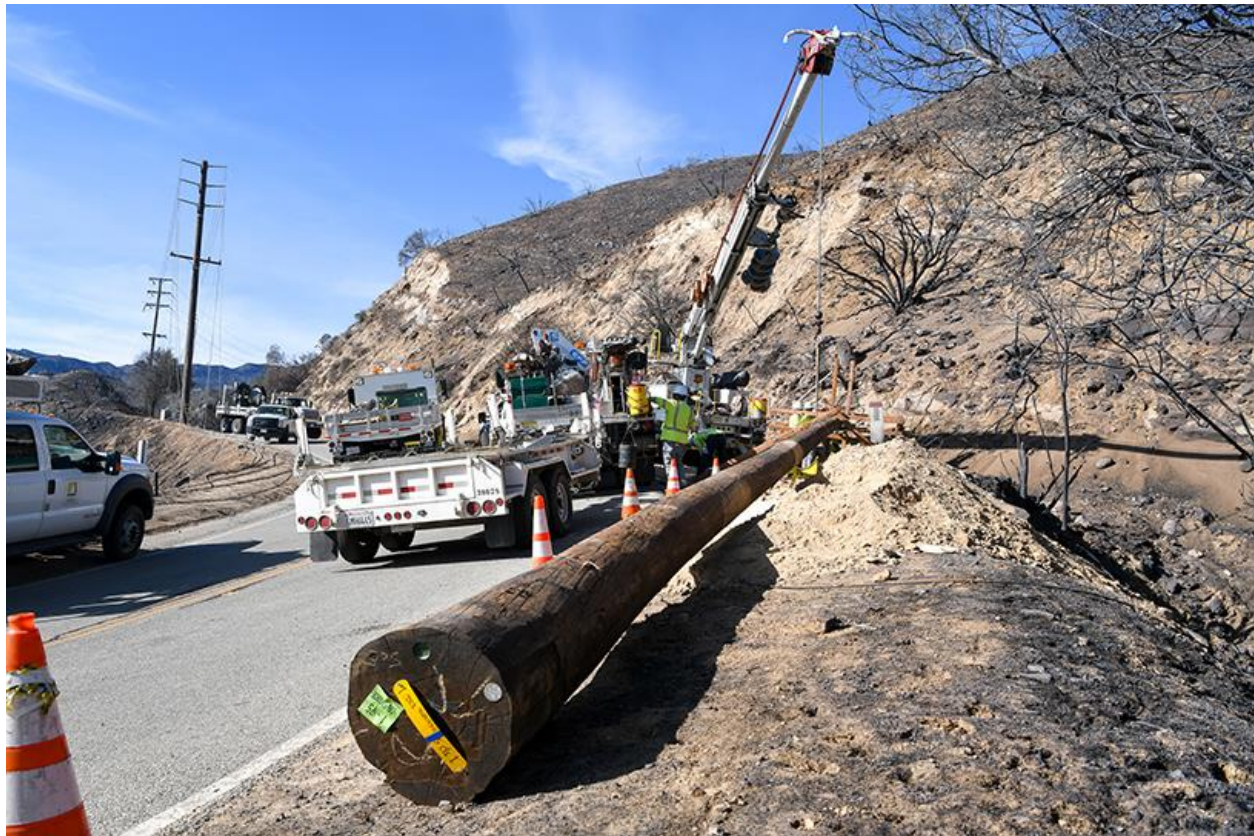
Figure 4—Infrastructure Damage – Power Pole
