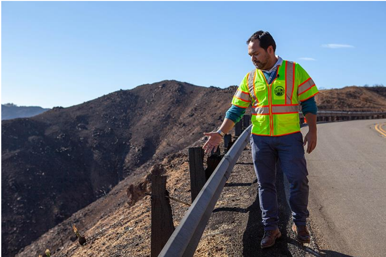
Figure 5—Infrastructure Damage – Canyon Road
