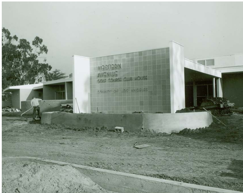
Figure 20. Construction of Clubhouse (1965), Chester Washington Golf Course SOURCE: Los Angeles County Department of Public Works, 1965
