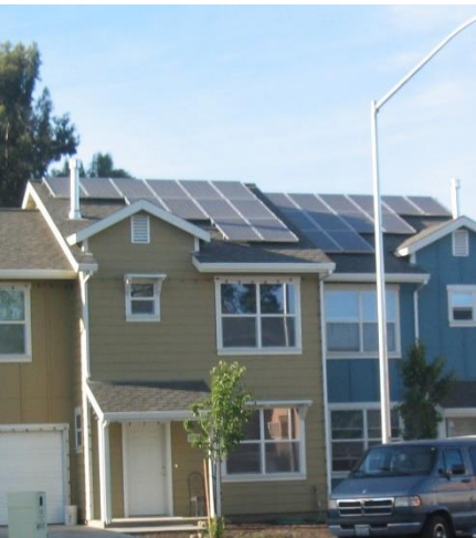
Example roof-mounted solar collector panels.
