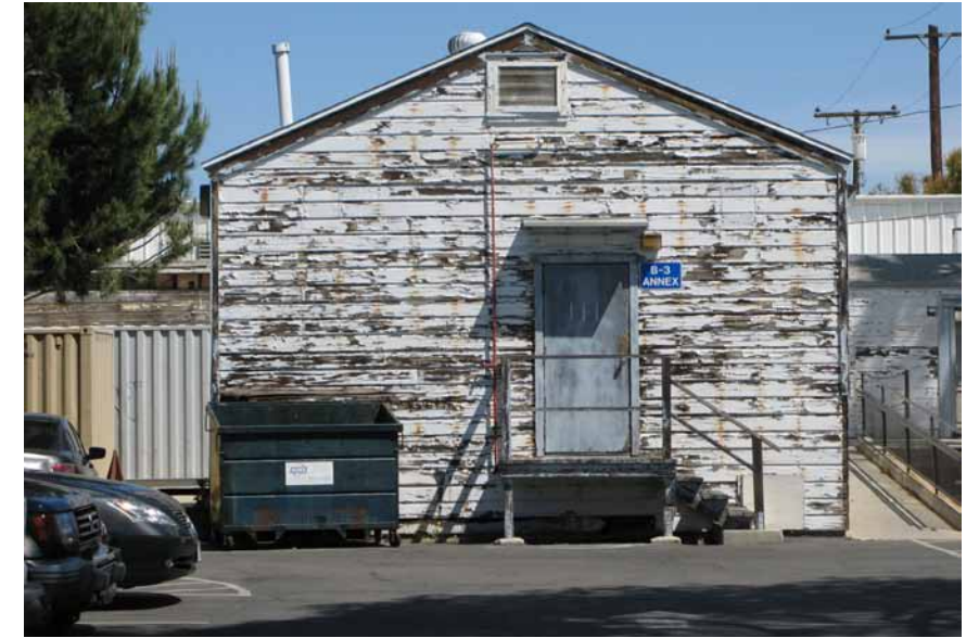
B-3 Annex - WWII Buildings in disrepair
