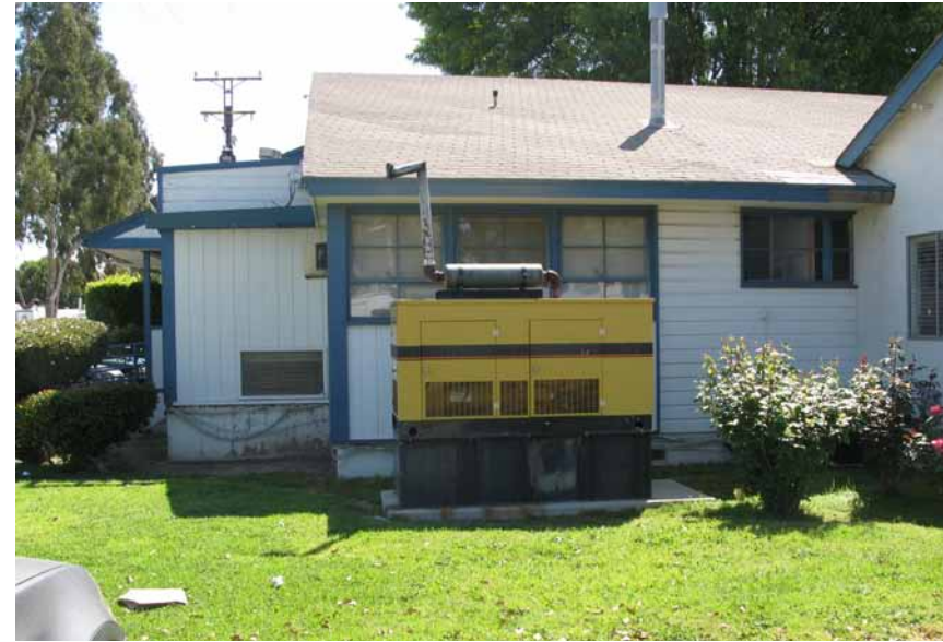
Existing interface with mechanical systems and modular buildings
