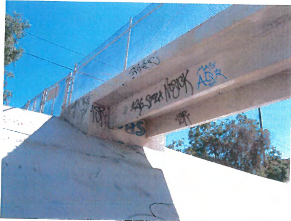
GRAFFITI IN CHANNEL - BEFORE
