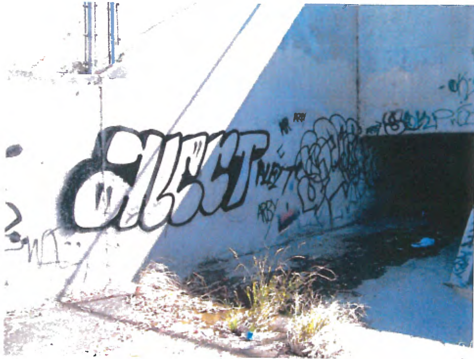
GRAFFITI IN CHANNEL - BEFORE
