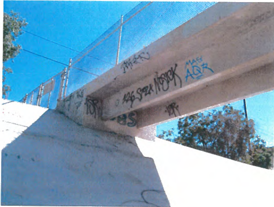
GRAFFITI IN CHANNEL - BEFORE
