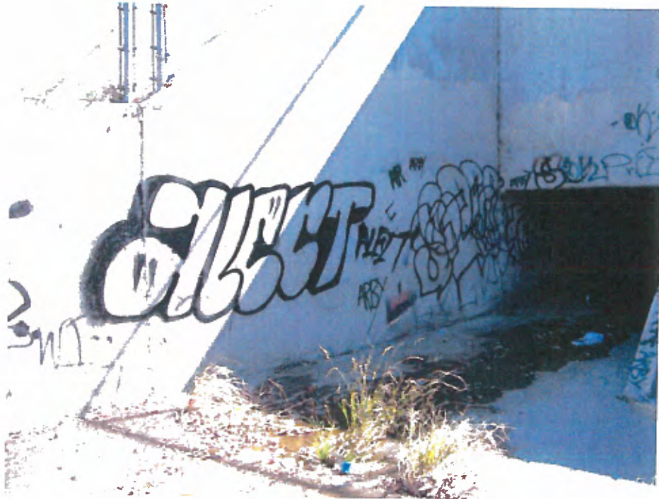
GRAFFITI IN CHANNEL - BEFORE
