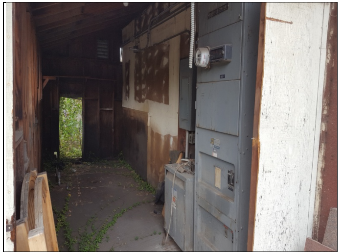
22. Electrical panel and dry transformer in empty structure.
