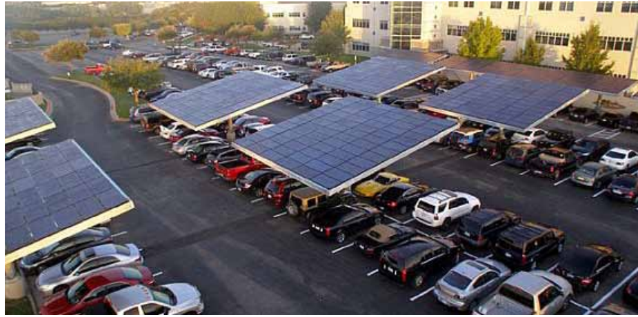
Photovoltaic panels shading parking areas
