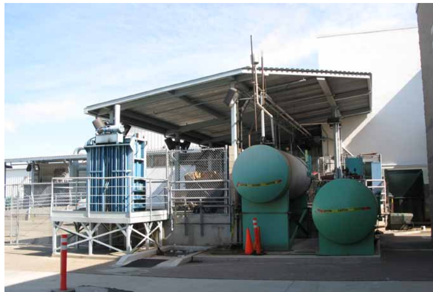
Central plant equipment
