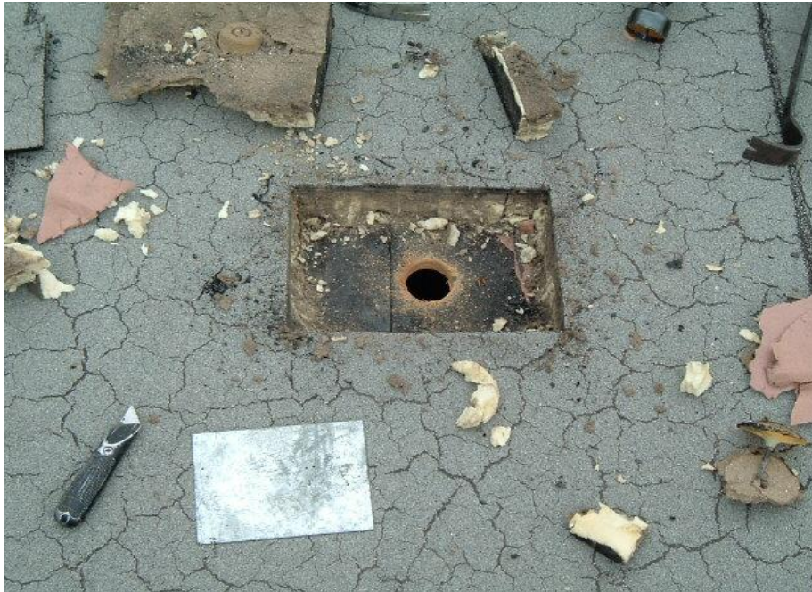
(3) Existing roof has one inch of insulation. The new roof will have five inches of insulation and a white roof.
