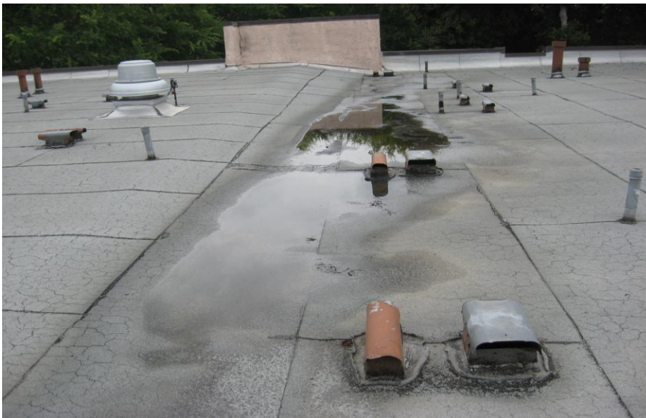
(4) Notice ponding, the new roofs will correct slopes to drain properly .
