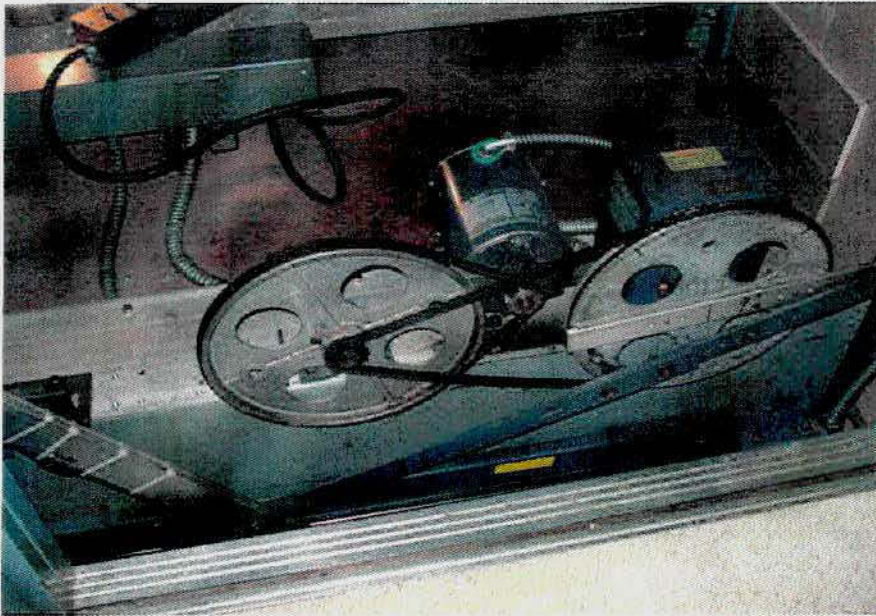
Door closing and opening mechanism worn out and out of date.
