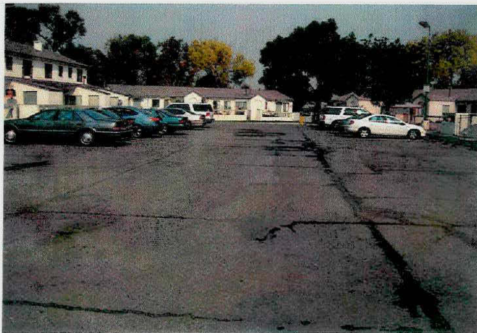
Cracking and general wear and tear
