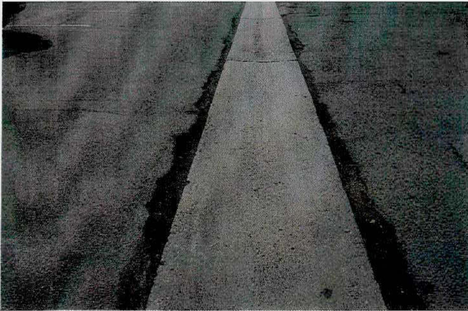
Major cracking and deterioration
