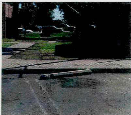
Broken wheel stops
