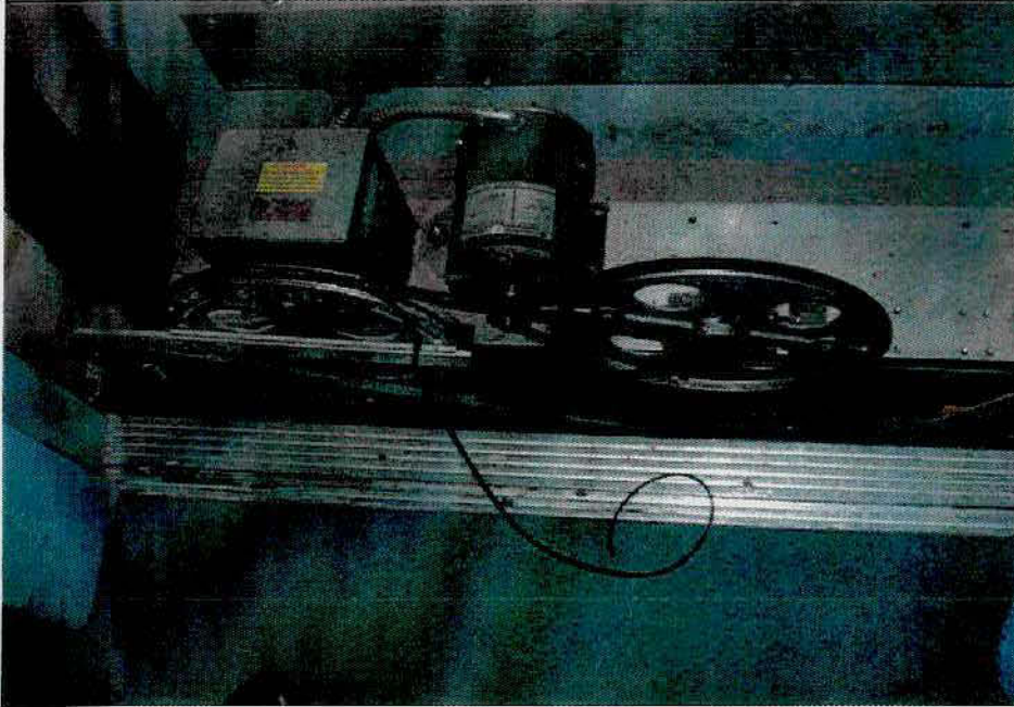
Worn out sheave is obsolete
