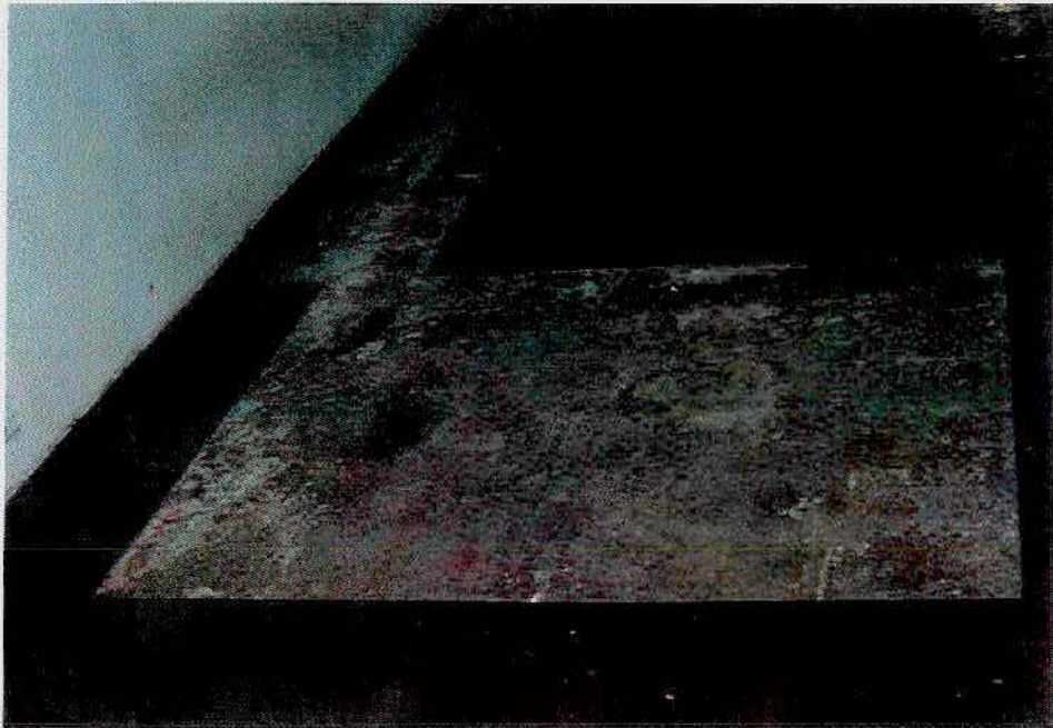
Ground floor internal breezeways - removing tiles which are delaminating due to ground moisture. Concrete will be cleaned and refinished.
