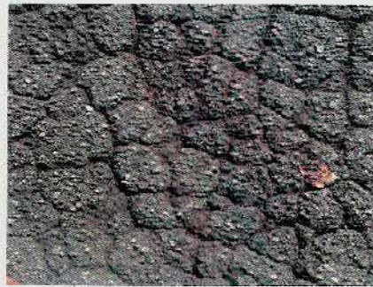
Severe cracking & deterioration
