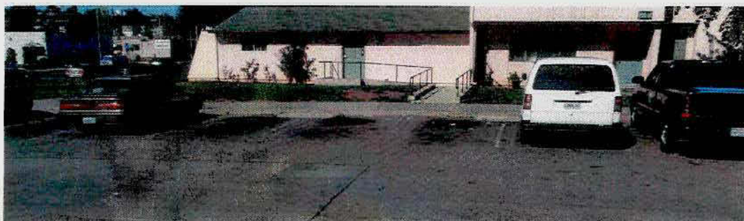
Pinos Parking Area - excess oil
