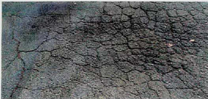
Severe cracking & deterioration
