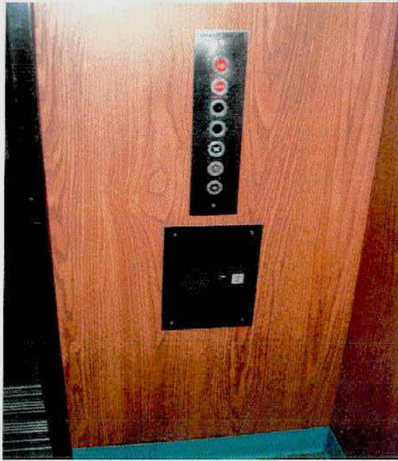
Controls not in compliance with Americans with Disabilities Act (ADA)
