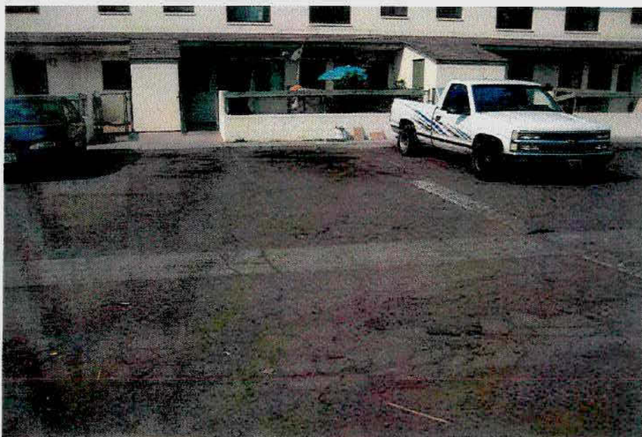
Severe Cracking & excess oil
