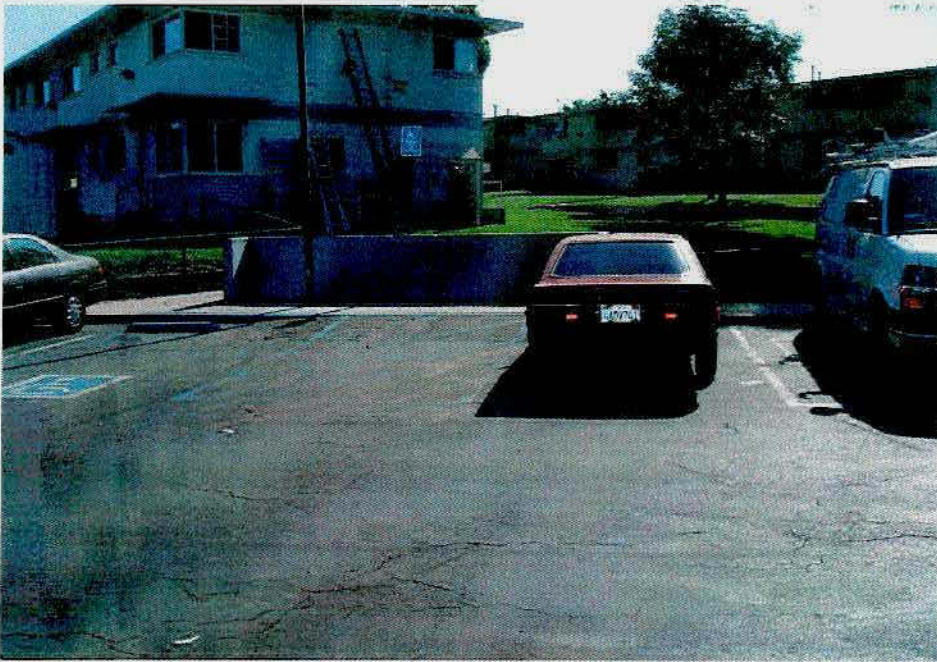
Cracking, faded striping, general wear and tear
