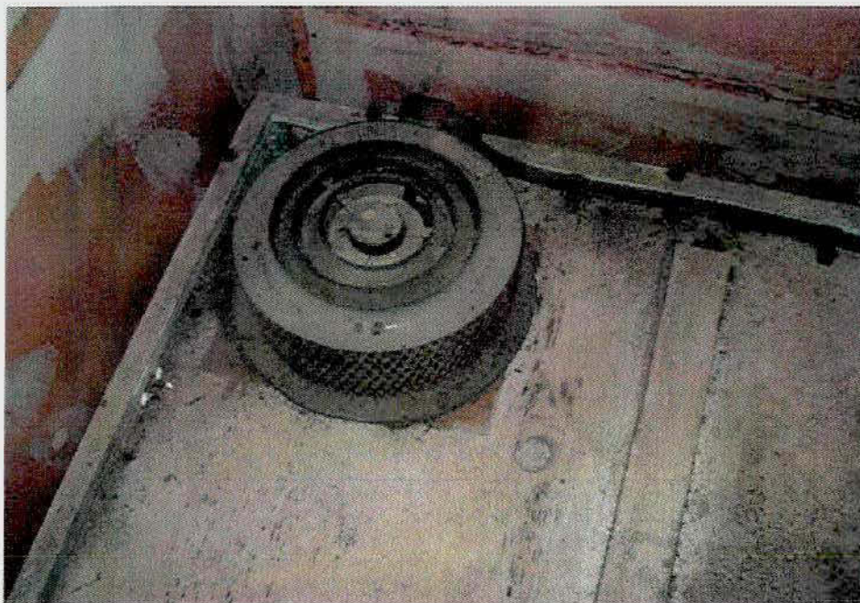
Air exhaust system worn and under performing
