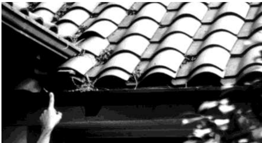
Fig. 15. Open ends of tile roofs may allow bat entry and provide roosting sites.
